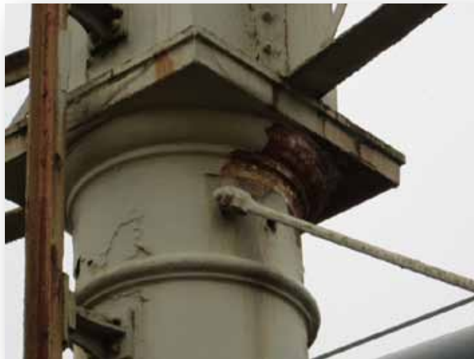
Photograph 13 Broken tie-rod bracket
