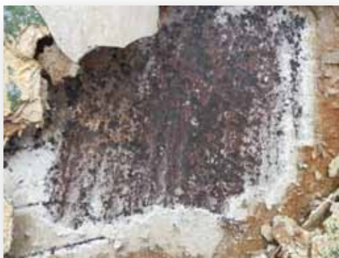
Photograph 20 Paint breakdown and condition of exposed structure.
