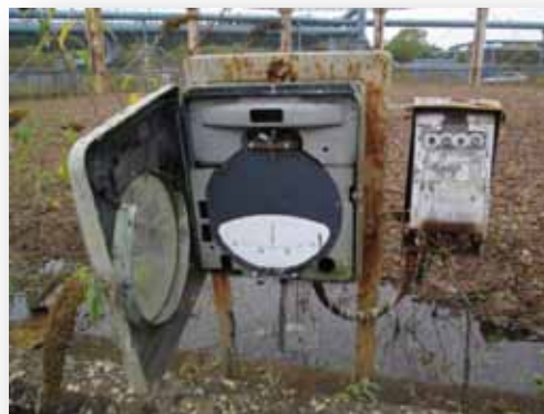
Photograph 19 Redundant "Kent" height gauge
