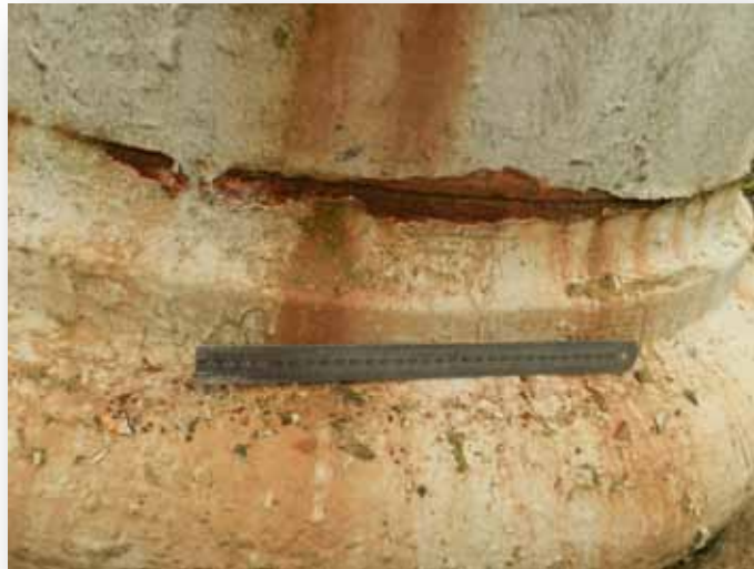
Photograph 22 Paint breakdown at joint
