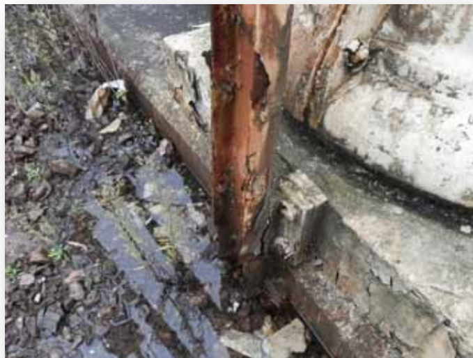
Photograph 23 Corrosion at bottom of guide rail
