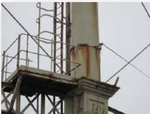
Photograph 16 Man access platform
