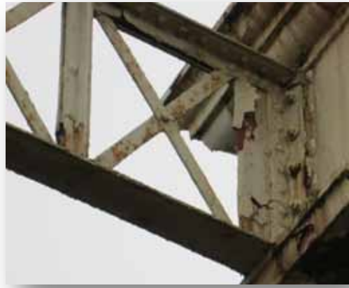
Photograph 12 Deformation of girder at attachment to entablature
