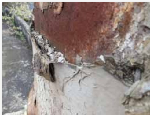
Photograph 21 Typical example of paint breakdown
