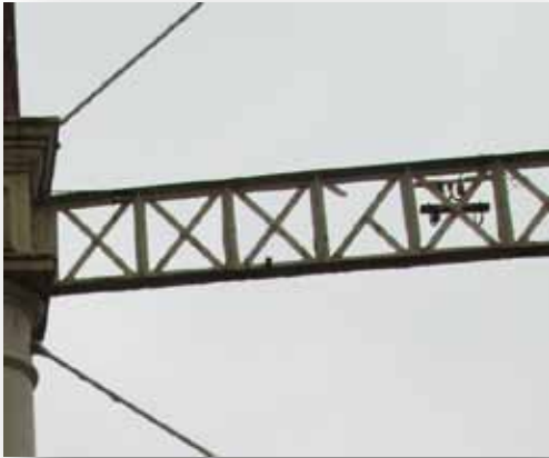
Photograph 11 Missing diagonal brace bar
