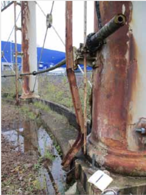
Photograph 14 Damaged roller guide
