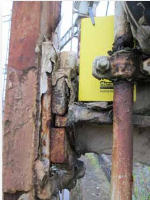
Photograph 15 Damaged guide bracket
